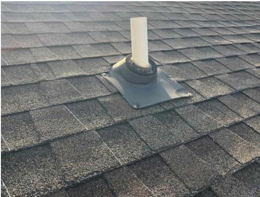
This pipe jack was installed backwards.
