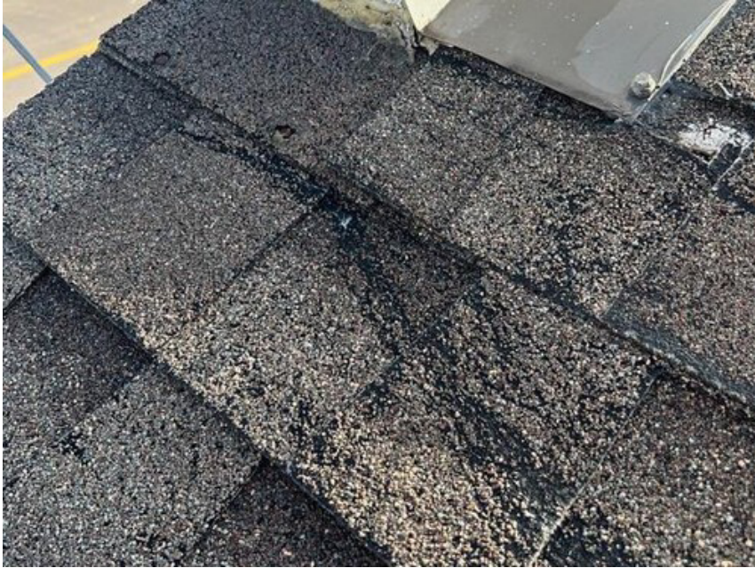
This picture shows wind damage to the shingles.
